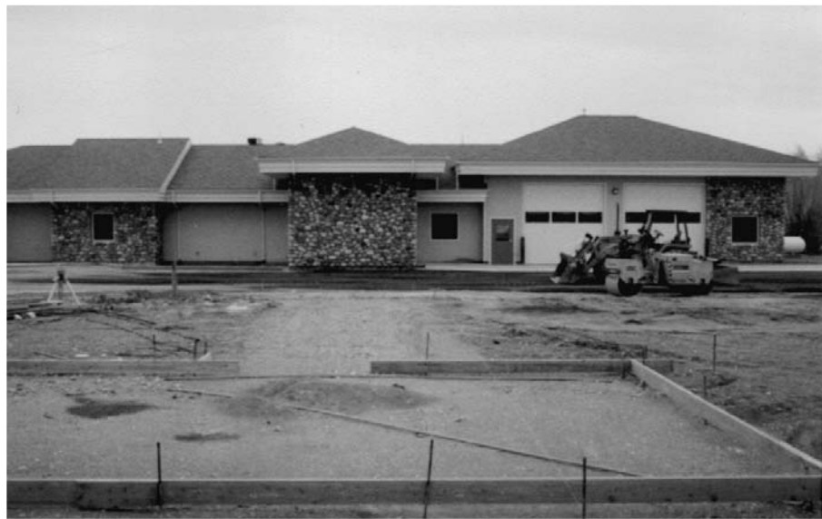
This clinic in Fairfield, built by the Camas Medical Services Board, has been assisted twice by ICF—once in 1993 with an initial planning grant and again in 1999 with a grant from the Kissler Family Foundation, a supporting organization of the Idaho Community Foundation. The Kissler family established Norco, and has a special interest in supporting health care-related projects.
